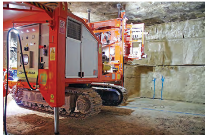
Automated cutting machine sawing a horizontal slot in the face – the bottom slot has already been cut. The operator’s position is on the left with the computer screen
